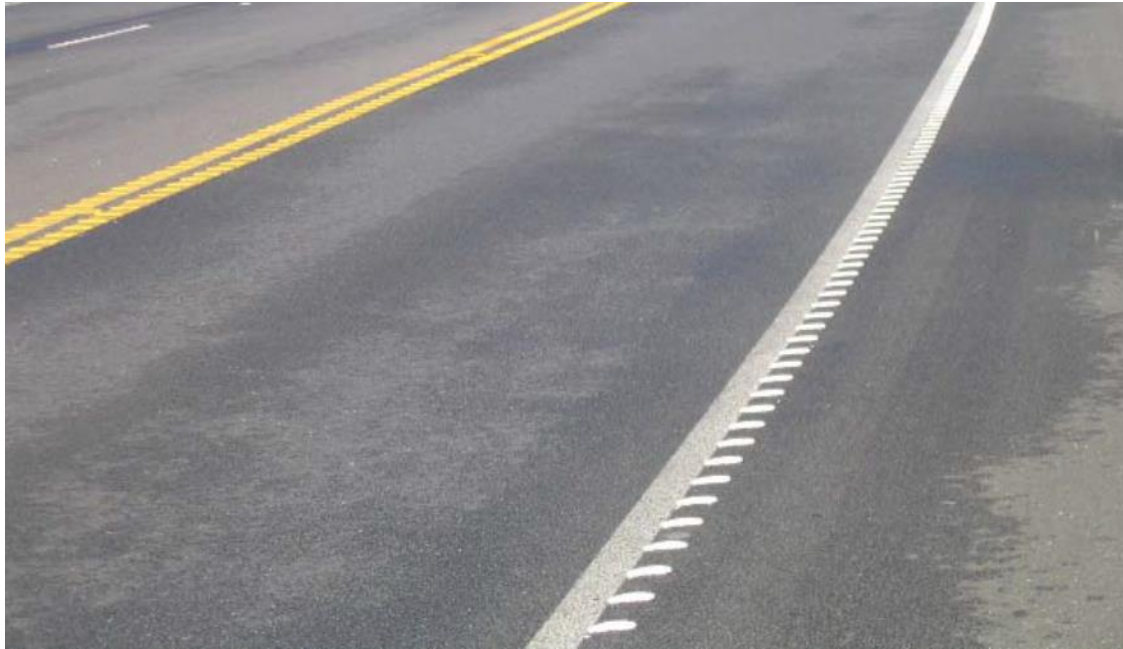
Top photo: Milled-in rumble strip on Highway 16, Sacramento County. Photo by John Swann
